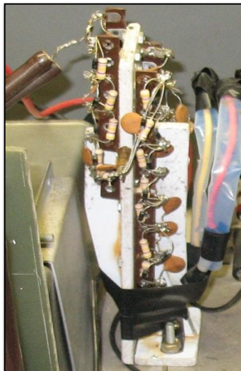
Picture 2 — Closeup of the diode strings.
