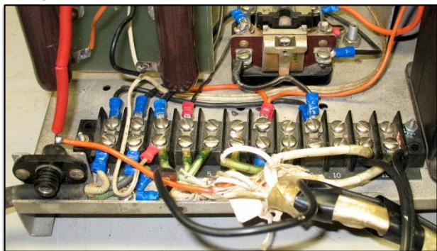
Picture 1 — The new terminal strip. Not a big deal but all the wires, except the white ones, the cable to the amp, were either cut or missing. Fortunately, I got a manual with the amp and a few minutes with the schematic showed how everything should be connected.
